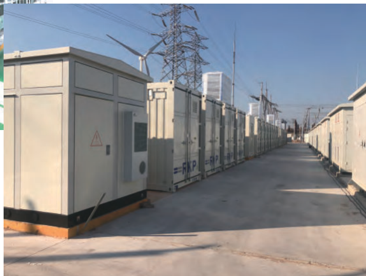
Figure2: The largest national 10 MW/40 MWh vanadium flow battery demonstration system
