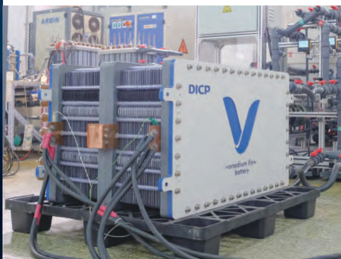
Figure3: New generation 30 kW vanadium flow battery stack
