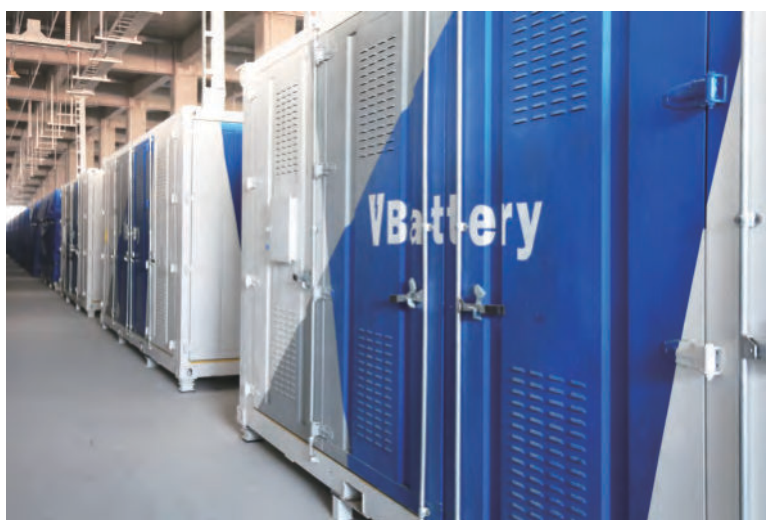
Figure4: 100 MW vanadium flow battery plant
