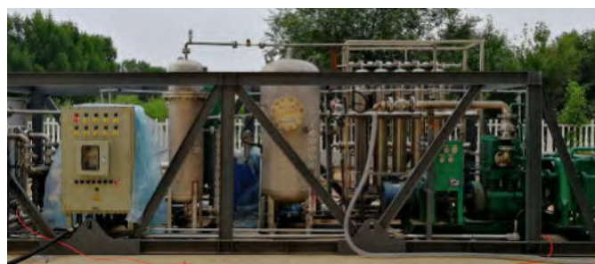
Figure 3: PTFE membrane contactor for biogas purification
